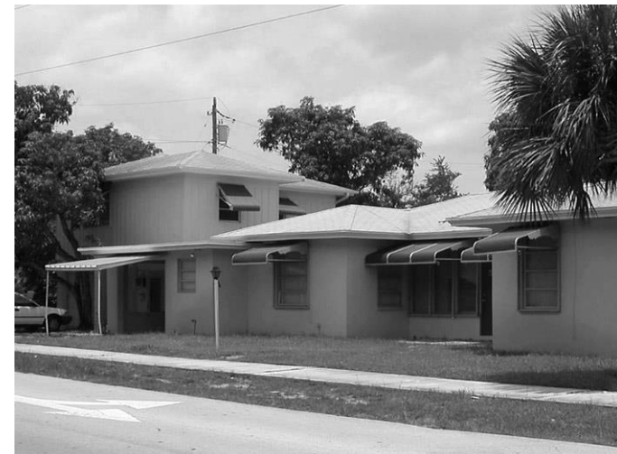
This building has stucco on the first story and wood siding on the second story.
