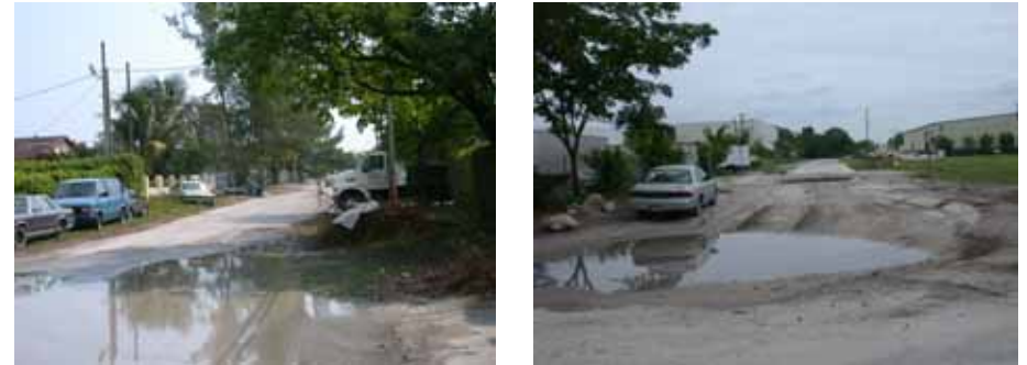
Figure 16 – Localized Street Flooding
