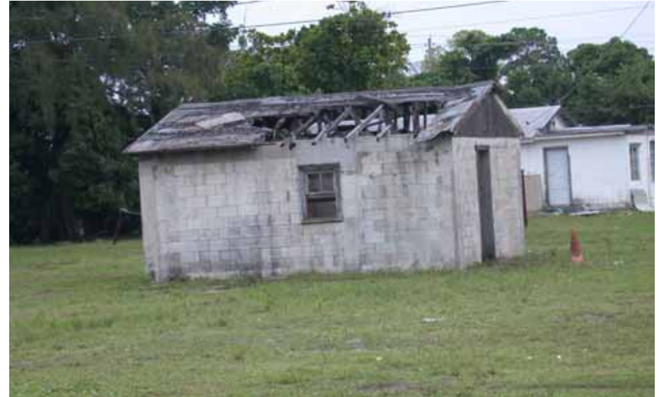
Figure 11 – This Dilapidated Building on Poinsettia Drive Should Be Removed.
