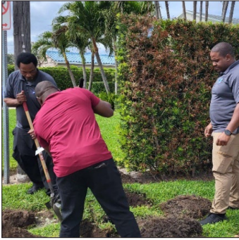
Locating dual check on water meter
