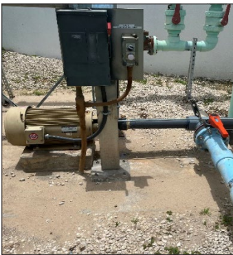
New pump and motor
