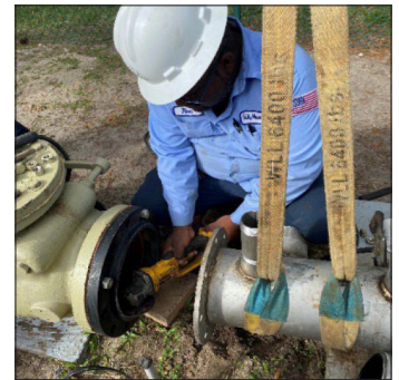
Raw Water Well 17 Flushing Port
