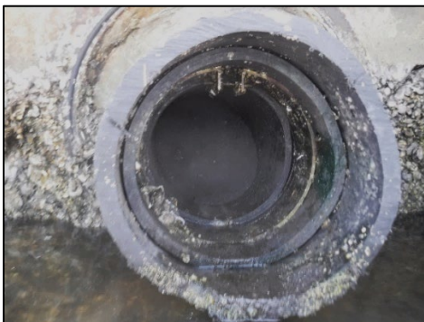
Inline Valve, Image courtesy of APTIM 2018.
